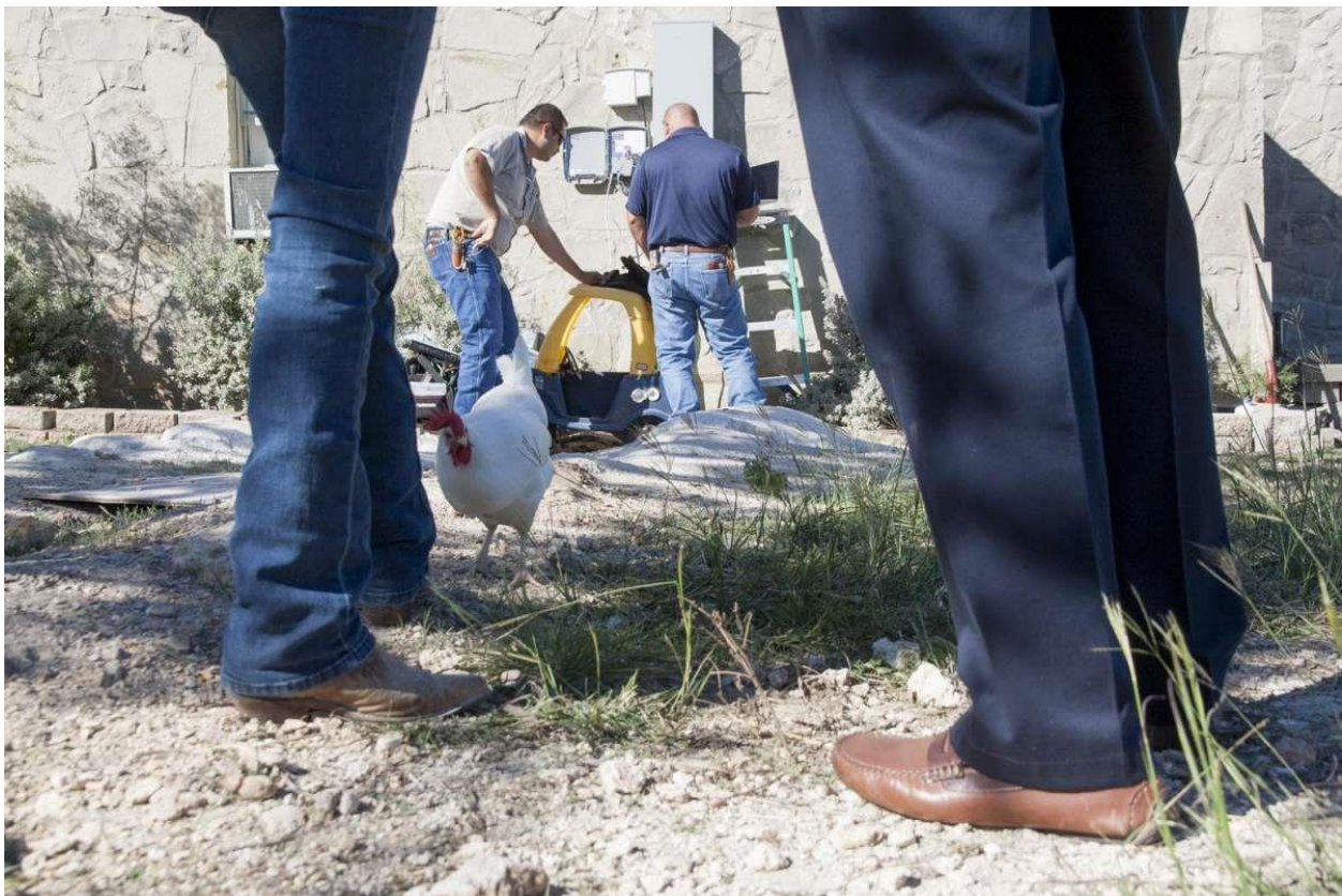
Telecommunications Technician Jonathan Zuniga and network engineer Wade Rust install the first GVTC gigabyte ultra-fast Internet service in the region Friday October 3, 2014 while Carol Steele and GVTC spokesman Bruce Forey watch. Photo Courtesy: Julysa Sosa, Freelancer / For the Express-News
